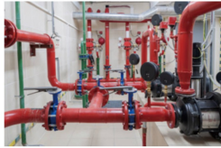
Airport and Subway Fire Protection System
