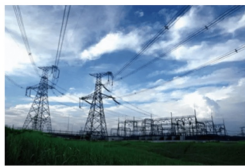
STATE GRID UHV SHANDONG RING NETWORK
