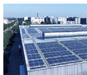
Solar Mounting System
