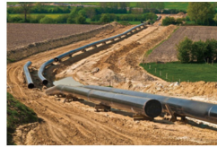
Oil and Gas Pipeline for Transportation
